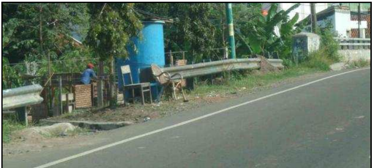
Broken Guard Rail by Local People for Their Access Road
