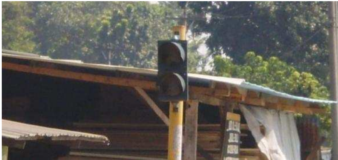
Traffic lights are not working and one pointing in wrong direction
