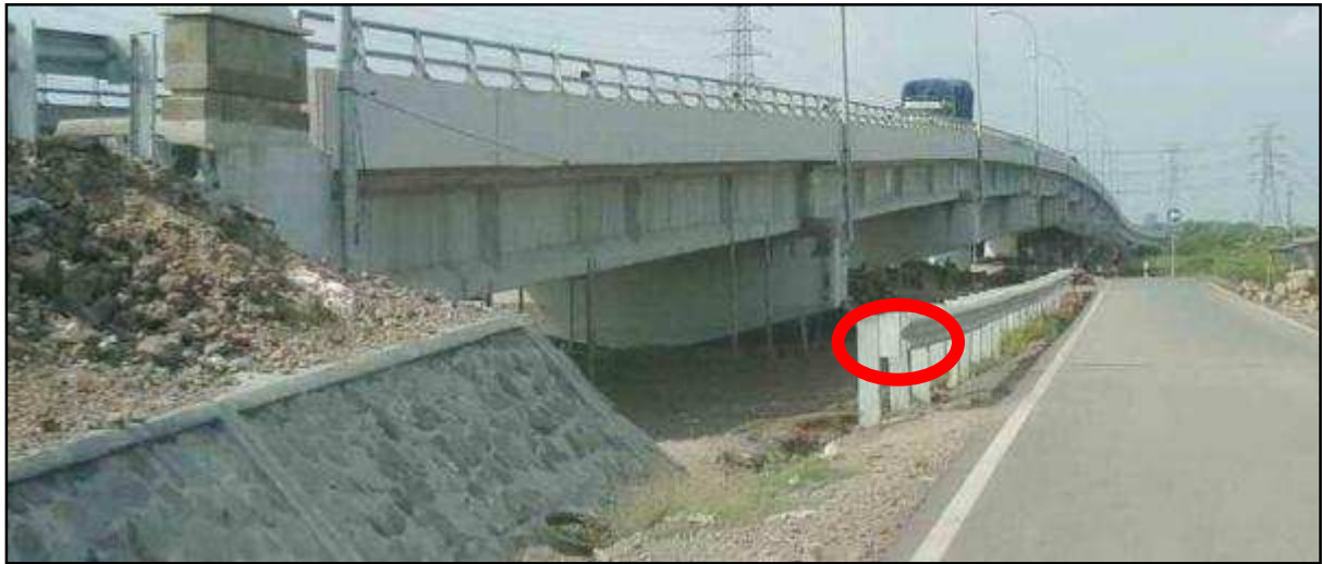
Exposed End of Guard Rail & Poor Signing, Circled (see below)
