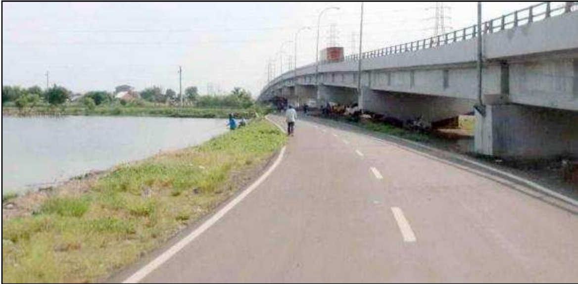
Local Road - Two Way - Lack of Guideposts or Guard Rail
