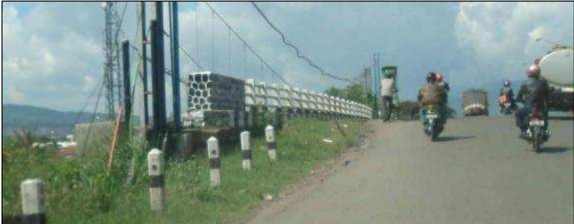
Potential hazard for road user, no guard rail approaching the bridge
