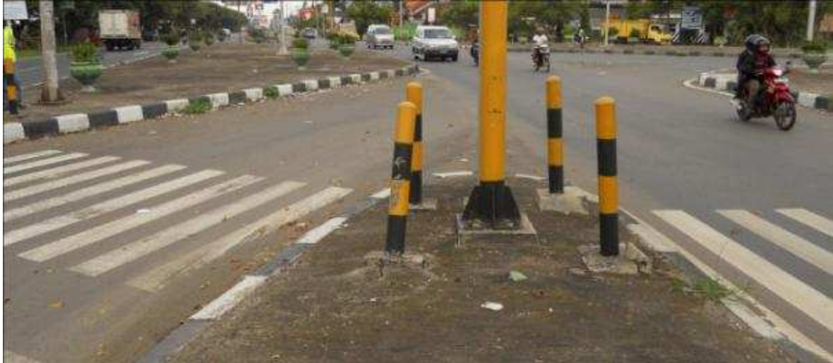
Blocked pedestrian crossing with signal light and crash protection poles
