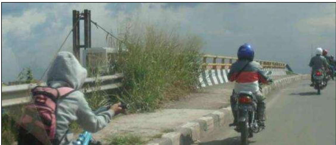
Better condition of guard rail but needs to have a solid/strong connected to parapet
